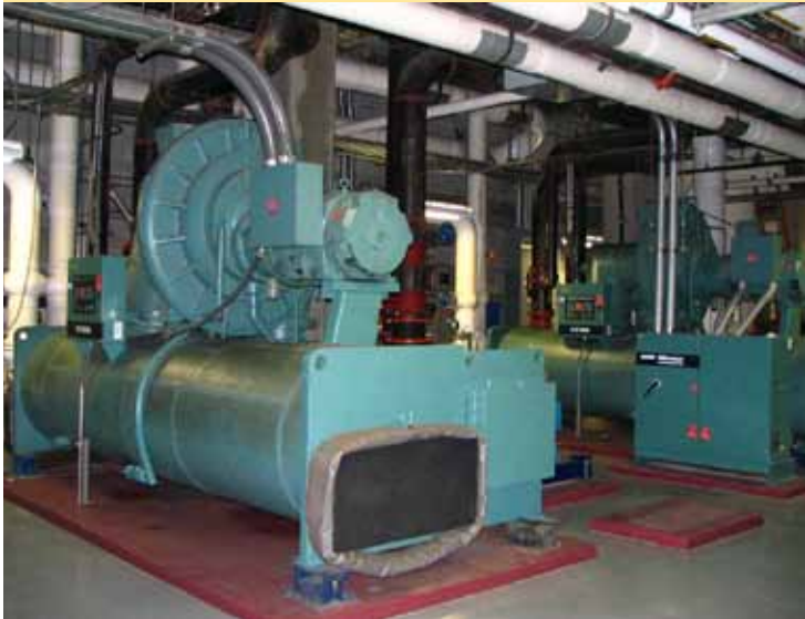
Variable speed drives and chilled water reset temperatures optimize chiller energy.
