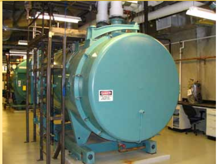
Boiler combustion optimization controls reduce fuel use.
