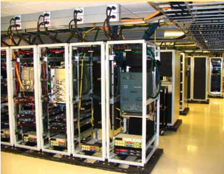
Heat recovered from server rooms is used to preheat laboratory supply air.
