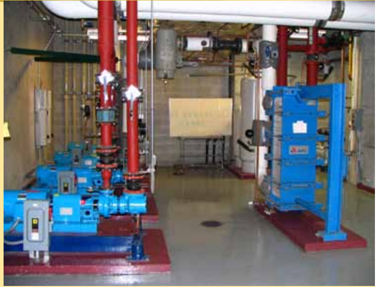
Waste heat from server rooms, environmental rooms and other heat sources is used to preheat buildings.
