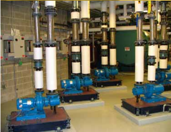
New and retrofit drives for hundreds of fan and pump motors reduce energy requirements and extend equipment life.
