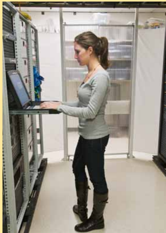
Delivering the coldest air from cooling equipment to server room cold aisles and isolating server cold aisles from hot maximizes the utilization of cooling energy.
