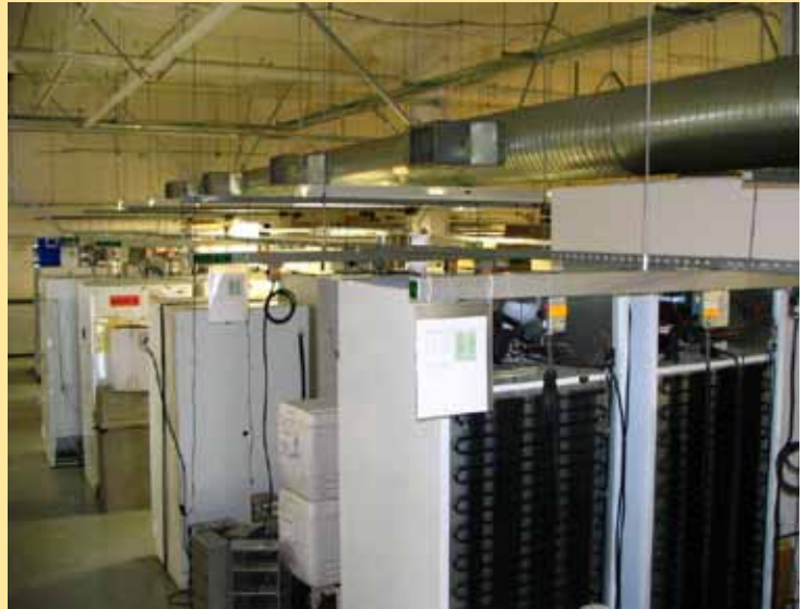
Use of outside air for 'free cooling' minimizes mechanical cooling.
