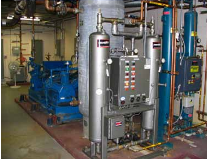
Highly efficient compressed air driers reduce use of compressed air.
