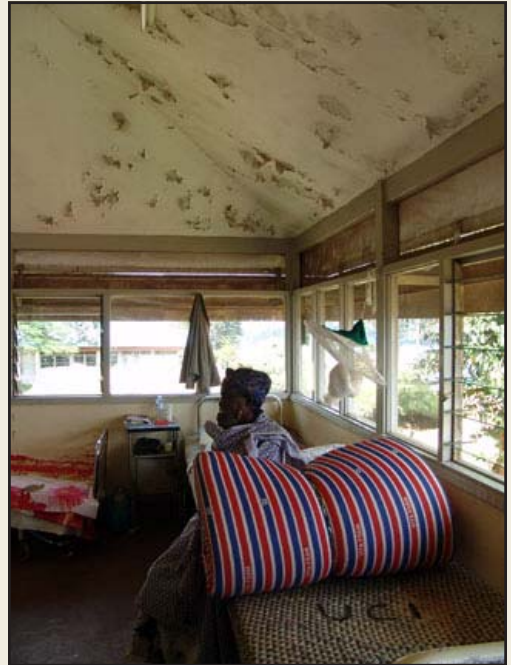
Crumbling ceilings and broken windows at the UCI
